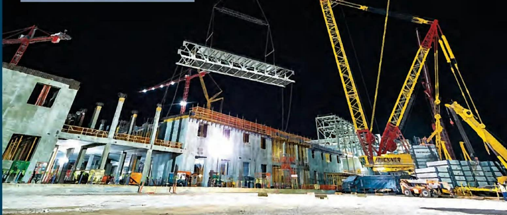
One of US crawler crane specialist Buckner's two Liebherr LR 13000 lattice boom giants
